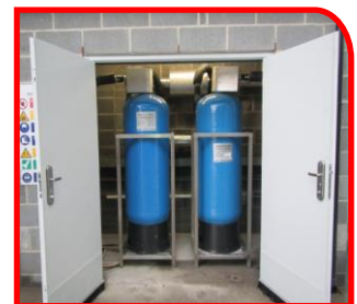
IHF Deionisers are installed in a purpose built extension
