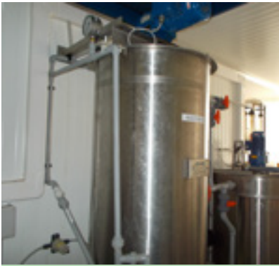
Struvia prototype reactor at the Brussels-North WWTP
