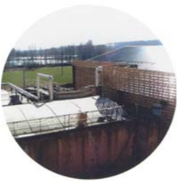
Luneville, France (2002) Simultaneous nitrification/denitrification after physical-chemical settling 4 cells, 63 m 2 each. 50 000 PE
